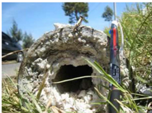
Fig. 5. Silica scaling in Dieng power plant, which is an obstacle of fluid flow [35].
