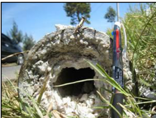
Fig. 1. Silica scaling in injection line.
